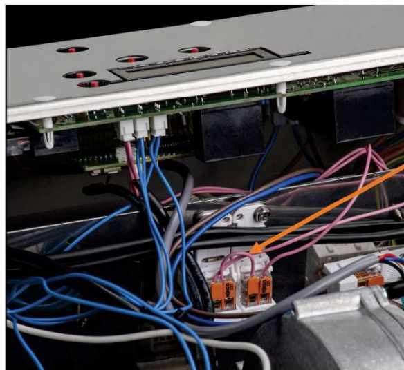
Looped Pink Wire – Fireman's switch connection
