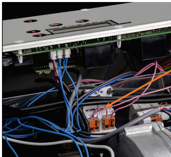
Looped Pink Wire – Fireman's switch connection
